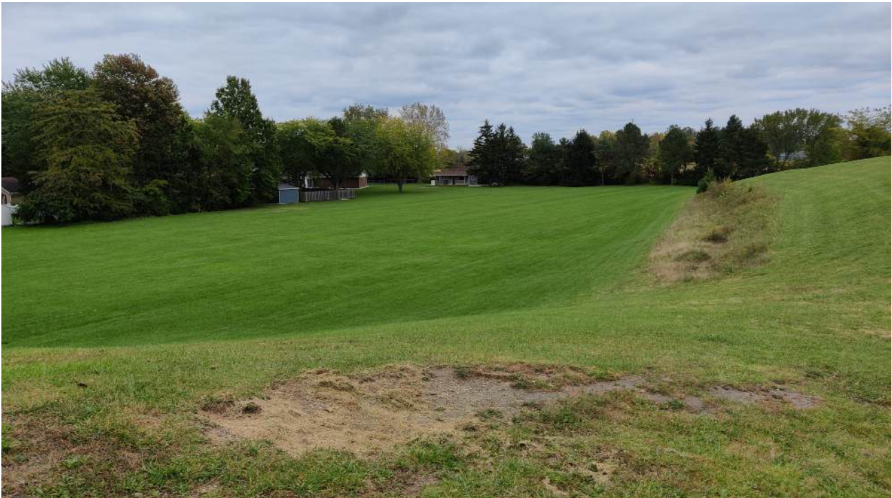
Drainage improvements needed at Portage Park
